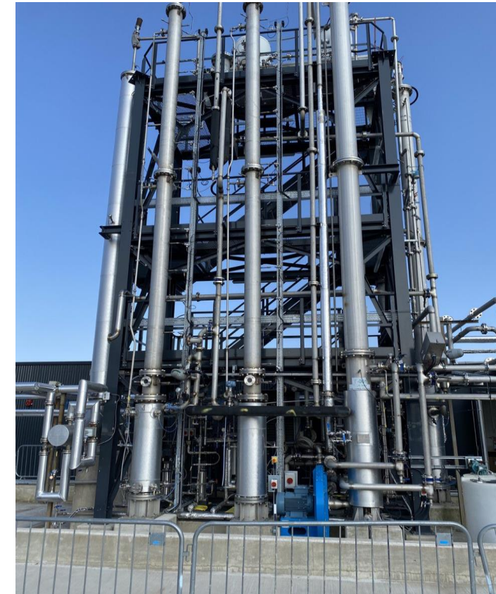
Our recent visit to the pilot scale amine solvent-based carbon capture plant at Translational Energy Research Centre (TERC) at Sheffield
